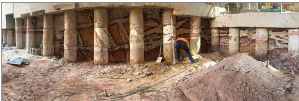
Figure 5: View from the first stage of excavation for a basement within the GPO Fault Zone ([6]).
